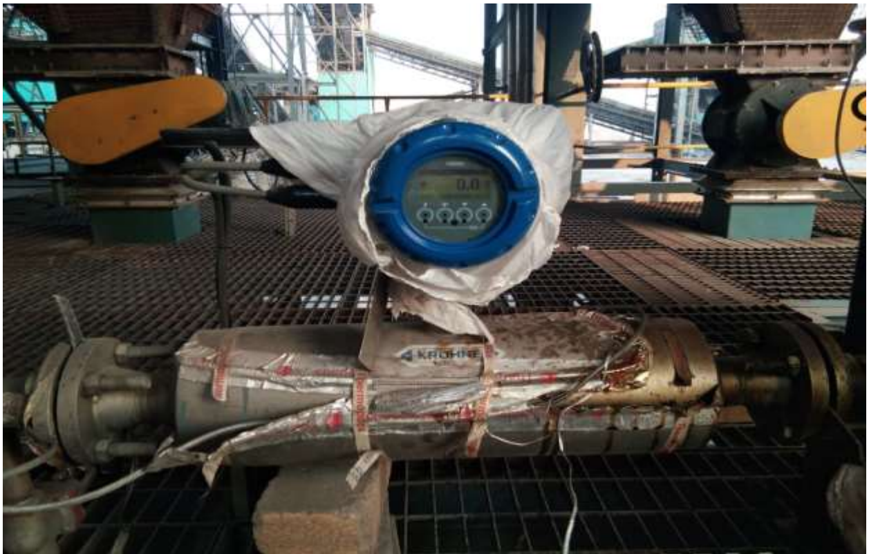
Concentrated spentwash flow meter
