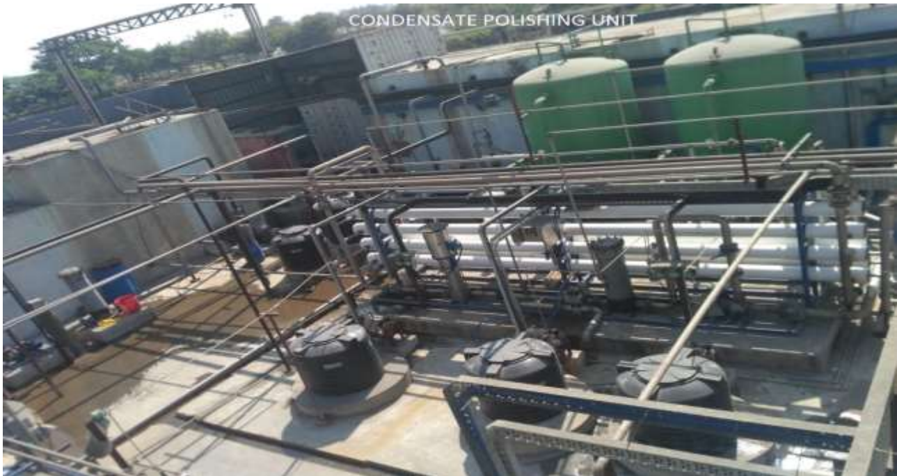
Condensate polishing unit
