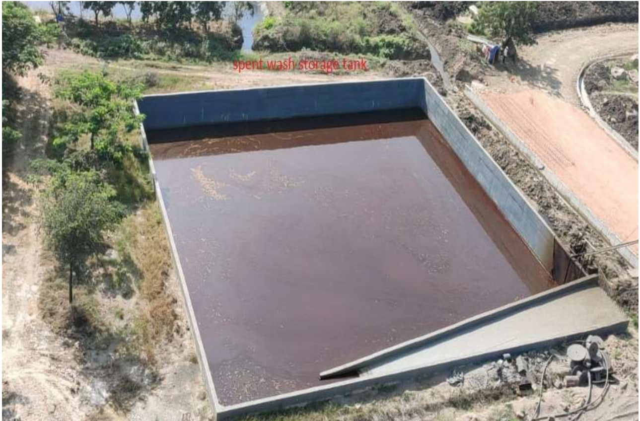
Spent wash storage tank
